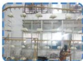
Painting production lines on the 1st Floor
