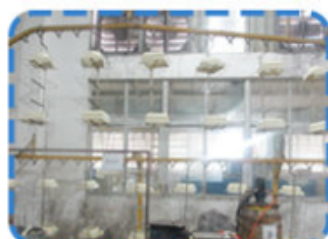
Painting production lines on the 1st Floor
